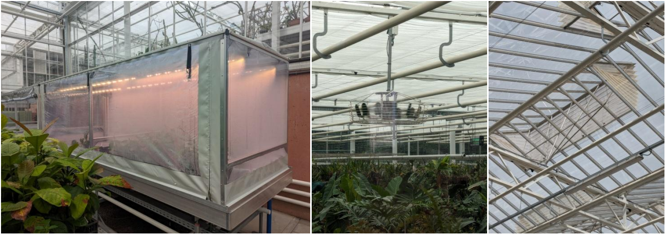
Nursery tech highlights: propagation tent, fans and netted vents
